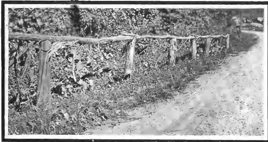
Old-style fences such as this one are out of place on the modern road and dangerous to traffic
